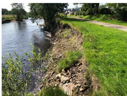
View of downstream right bank erosion from right hand bank
